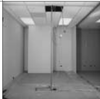
8. Flexible prewired electrical components can also be installed through ceiling runner prior to erecting any panels..
