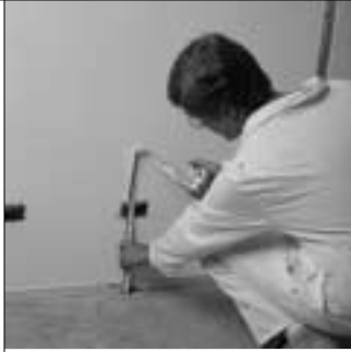
19. Measurements must be taken for openings to be cut in panels receiving electrical boxes.
