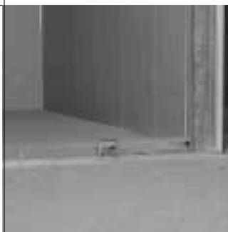
17. ...in sill area of glazed opening.
