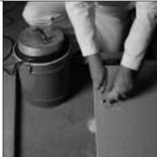
23. When cutting openings in fabric-covered panels, be sure to prevent gypsum dust from getting into pores of material.
